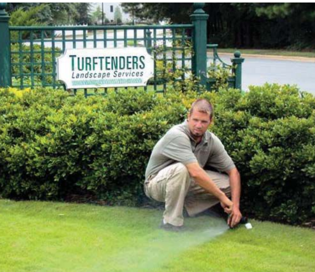
At left: Josh DeMoll, irrigation technician, sets an irrigation head. Below: A Turftenders' account undergoes an irrigation audit.
