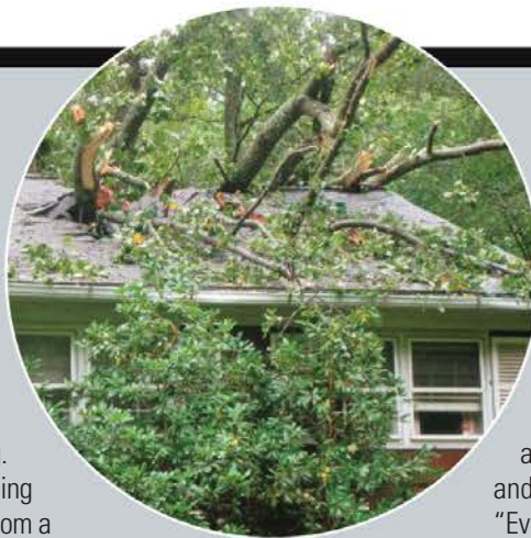
A tree smashed through the roof of a home in Trumbull, CT, near Stamford.
