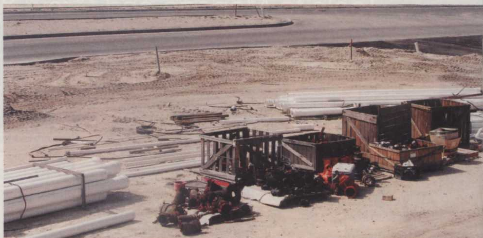
A Hoover Pump Station will supply 2,100 gpm of water to homes and common areas.
