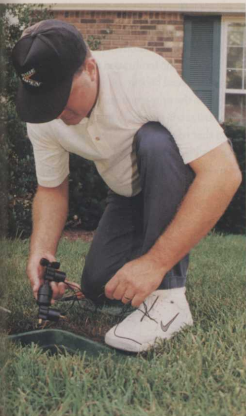
Installation and maintenance of residential fertigation systems is relatively simple.
