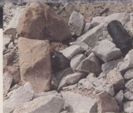
Debris like this is becoming an increasingly common problem at job sites.
