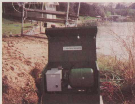
This 7.5-hp pump station distinguishes between high-flow and low-flow pressure demands.
