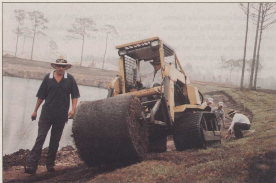
A Posi-Track crawler conquered the landfill's 3-to-1 slope and saved more than 1,000 hours of handwork as it laid big-roll sod over a towering Florida landfill.
