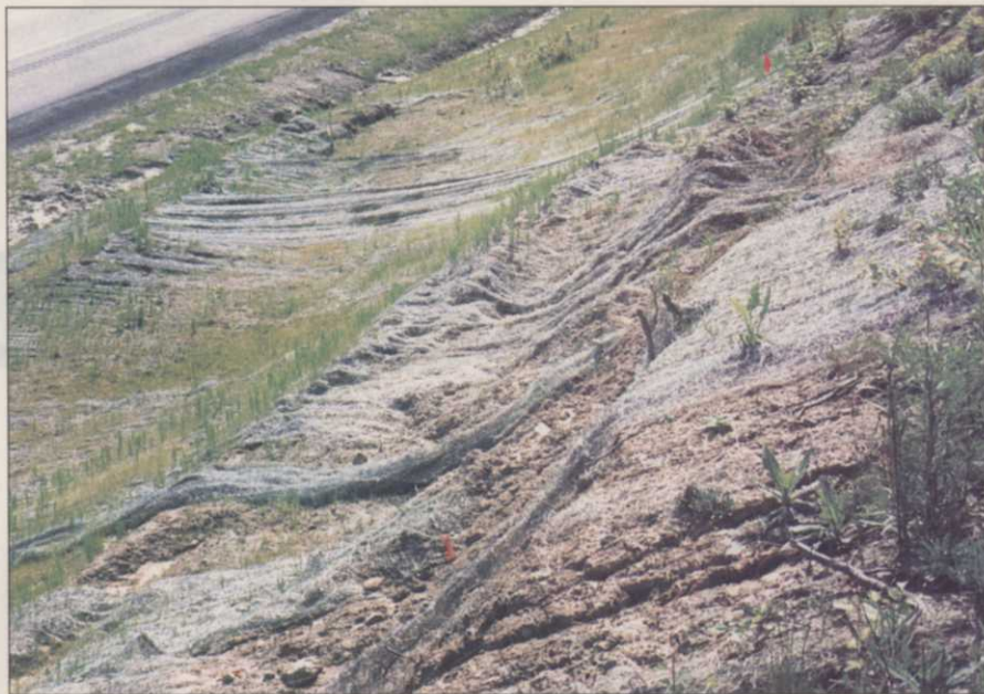
Correct installation of materials is essential for successful control of soil erosion. Heavy spring rains devastated this newly planted roadside even though a fabric covered it.
