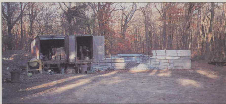
The staging area, where irrigation construction materials are held for use. Keep it organized.
