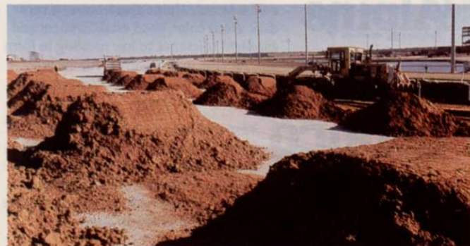
TurfGrids, fibrillated poly fibers, blended into this 80/20 planting medium provide stability to the bermudagrass racing surface.
