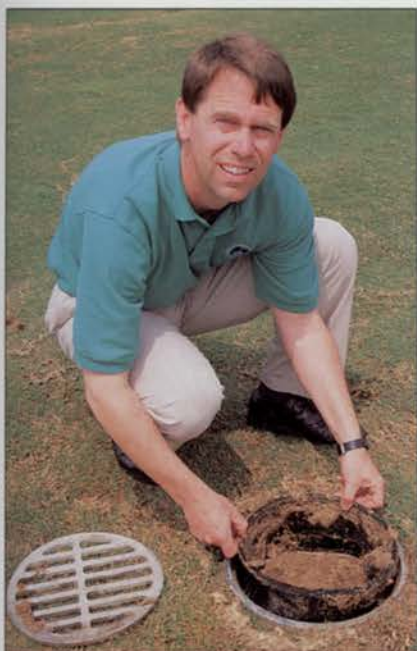
The siphons are one-foot diameter basins with grates to remove surface water.
