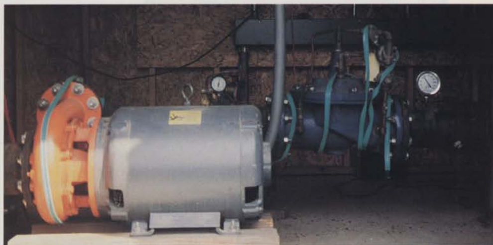
Steve Morton and his crew at Mallard Creek saved about $20,000 when they designed and installed this pump station.
