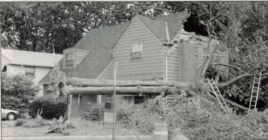
The owner of this house in the Cleveland area wasn't very happy with a tree that succumbed to high winds earlier this year.
