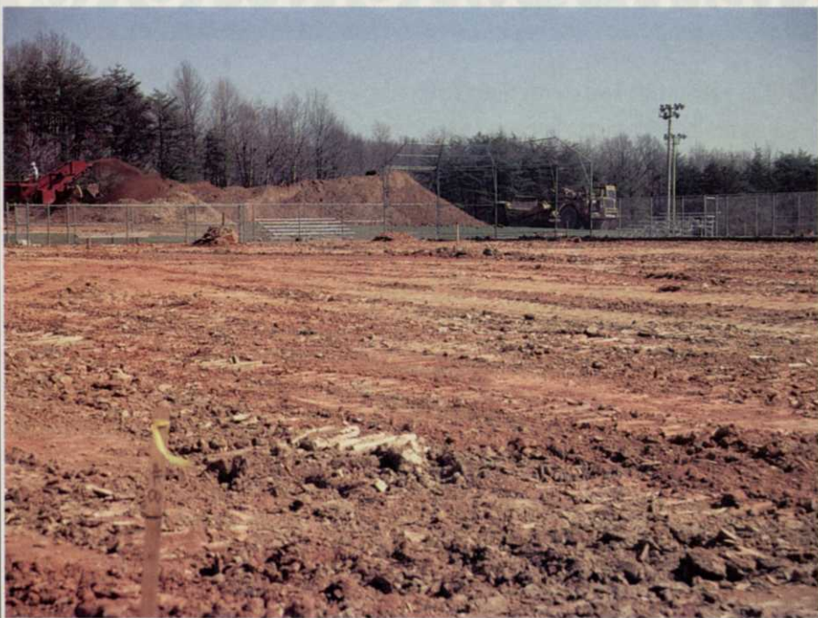
An athletic field after stripping and stockpiling of topsoil shows promise for the future.
