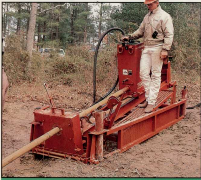
A whole new class of trenchless technology from Ditch Witch offers extended range with affordability.
