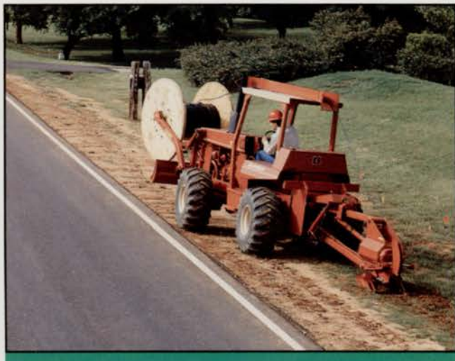
The Ditch Witch model 6510 equipped with the exclusive fiber optics cable handling system.
