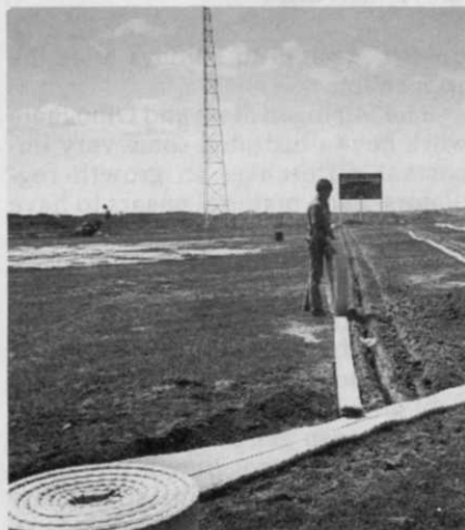
Installing the TerraFlow system laterals. The white areas are where turf was not able to survive because of high salt.
