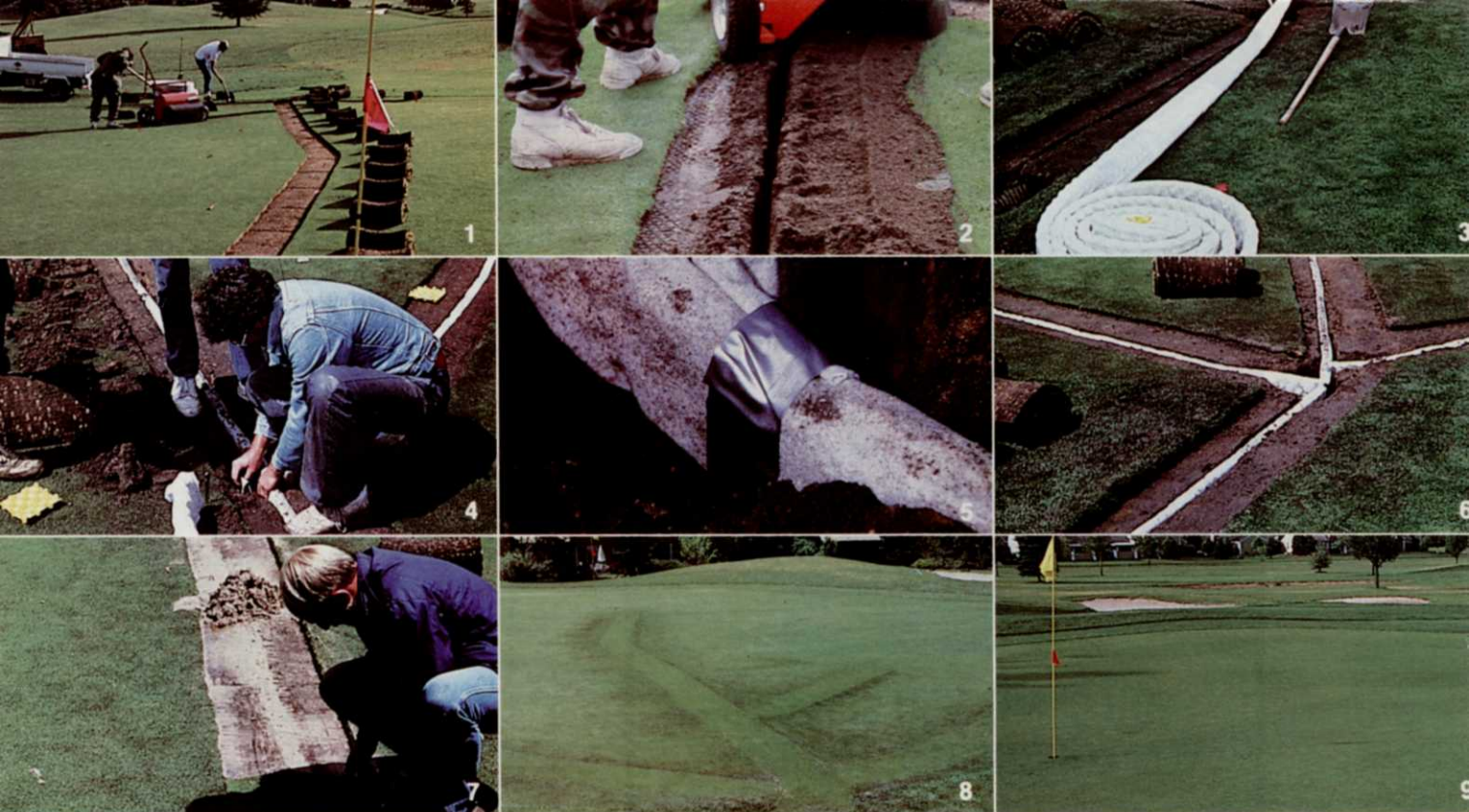
1. Rolling back sod where TerraFlow lines will run. 2. Cutting 2" wide trench. 3. Laying TerraFlow lines in 12" deep trench. 4, 5. Joining TerraFlow lines using only a utility knife and duct tape. 6. Fully installed TerraFlow System. Workers backfill with site soil, puddle with sand. 7. Replacing sod. 8. Completed TerraFlow System. Installation time: about 100 ft. per hour. 9. Green was back in play in 2 hours with TerraFlow. (Photos by Greg Fast, Turf Irrigation Supply, Englewood, Colorado.)
