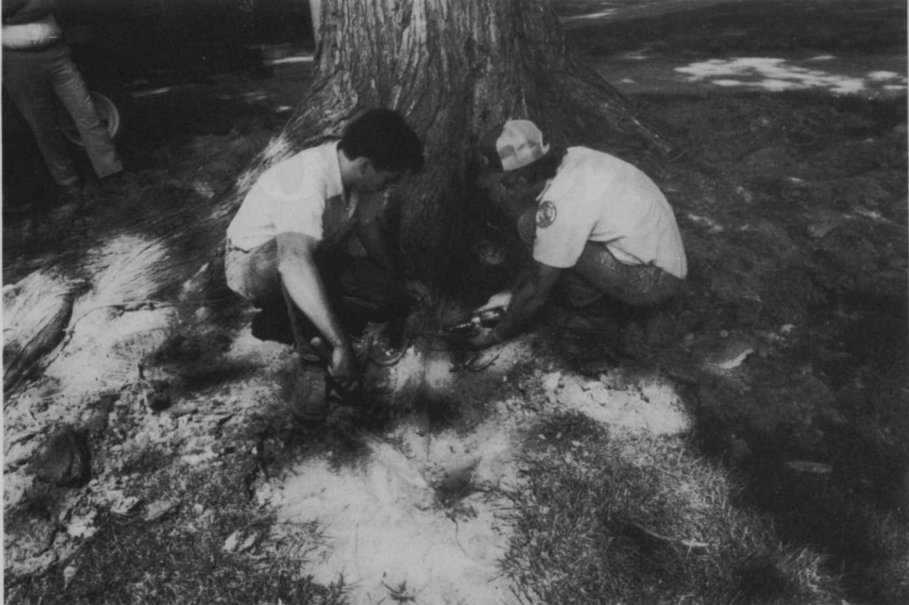
After soil has been removed to expose root flares all around the elm, university grounds crew members Douglas Lanham (right) and St. Clair McVicker drill holes and tap in injection tees. Tees are connected by tubing that connects to the tank containing fungicide mixed in the required amount of water. The fungicide is injected into the tree at 5-15 psi.
