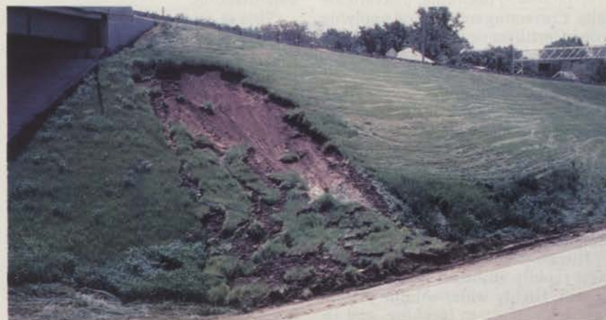
Studies have shown that low rates of water-insoluble nitrogen applied in the sodbed prior to laying sod encourages rapid root growth. A firm early knit of sod is important on erosion-prone cut and fill slopes along roadsides.
