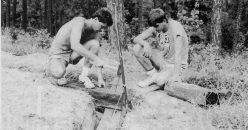
Students Blain Ritter and Jeff Etheridge work on the back retaining wall for the Sir Walter Raleigh Garden.
