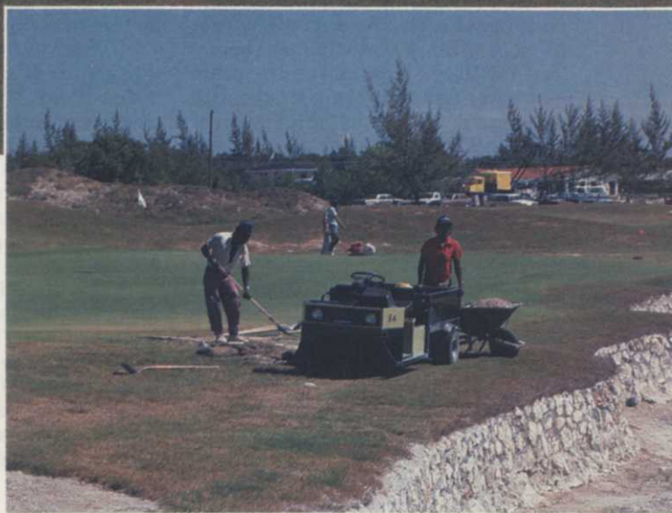
Mounds dominate the terrain at Britannia, reminiscent of Scottish courses, (top). $20,000 in brick support work, (bottom) stabilizes water hazards on the course.
