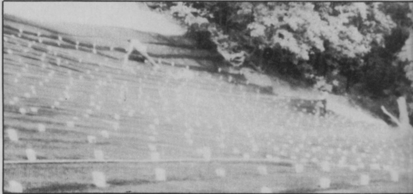
Enkamat pegged into Jersey Shore slows the Atlantic's erosion of the 200-ft. slope.
