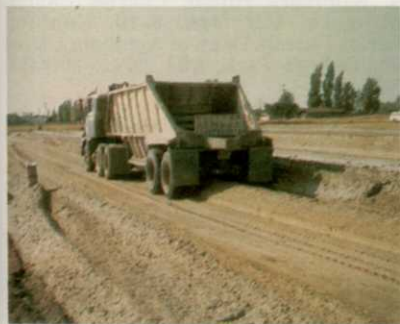
Sand base is layered over the entire field. This provides adequate drainage during fall rainy periods in most climates. Finished grade is flat and no crown is needed.
