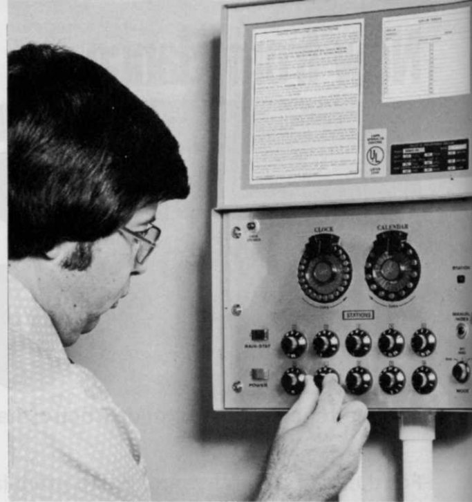
Typical controller operational panel.
