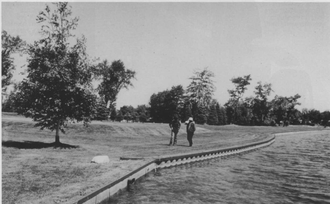
Corrugated sheets (lower left) show more wear even though they were installed after the piling (center).
