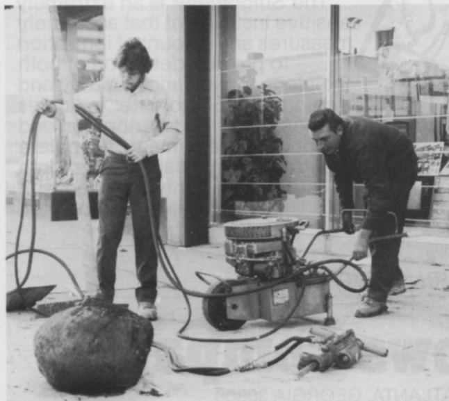
Two crew members prepare to chisel a hole through the sidewalk. The portable hydraulic unit is wheeled into position.
