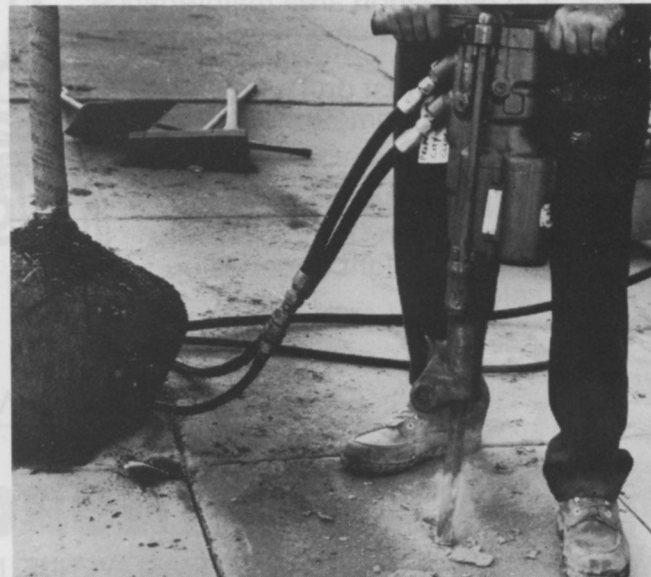
After the sidewalk has been scored and cut, the jackhammer is used to break-up the concrete.
