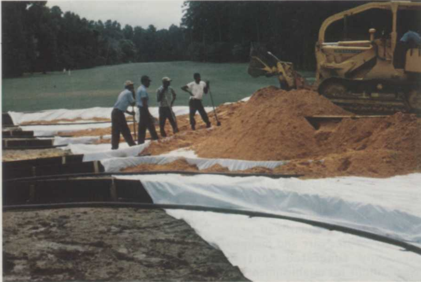
Spreading Sand over Tu-Tuf barrier on model green, 6 compartments, showing drainage pipes in each compartment.
