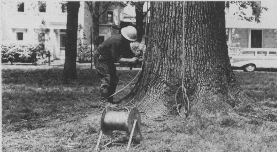
According to Code recommendations, two down-conductors are needed for large trees having trunks more than three feet in diameter. Cables lead from air terminals at top and on main branches to at least two grounds, located outside main root system.
