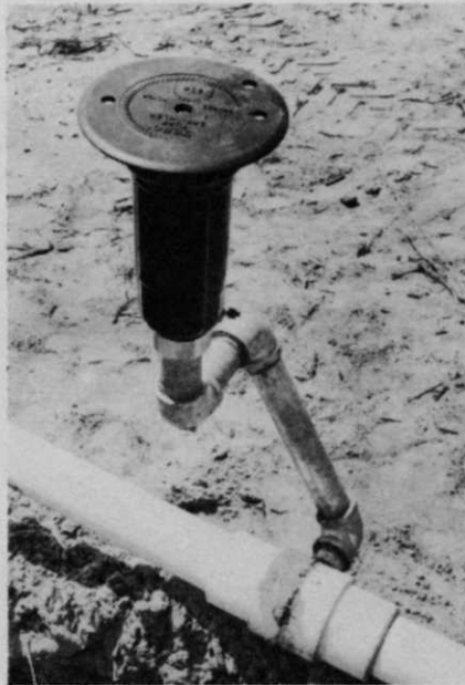
This system features individual head control, to allow for the different water needs of certain areas on the course.
