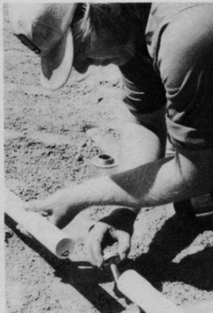
Solvent welds are completed in minutes. Interior of bell and end of one section is coated. Exterior of the spigot end is coated. Joining is done manually.
