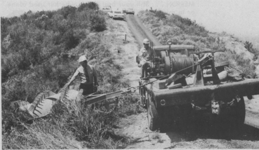
Developer, G. I. Morrow, inspects his invention, a unique brushroller. This picture, taken by the Los Angeles Department of Water and Power, shows that the modified spiked road compactor can pulverize and compress more than 8,000 sq. ft. of hillside brush an hour.
