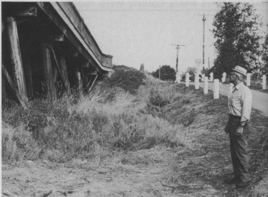
Semi-dormant weeds and grass at base of wooden viaduct shows where weeds and grass have been treated to hold back growth. Without chemical control this growth would be head-high by mid-summer.
