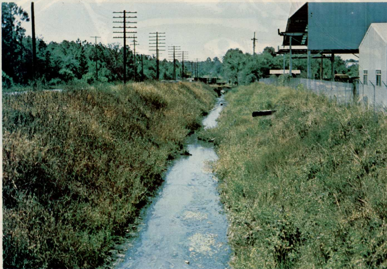
Clean main ditch has been kept free of brush by application of Ammate X two months after dragline operation. The ditch bottom, slopes and berm were sprayed. Dead vegetation has been removed allowing good water flow. Mowing will permit grasses to thrive on slopes and berms.
