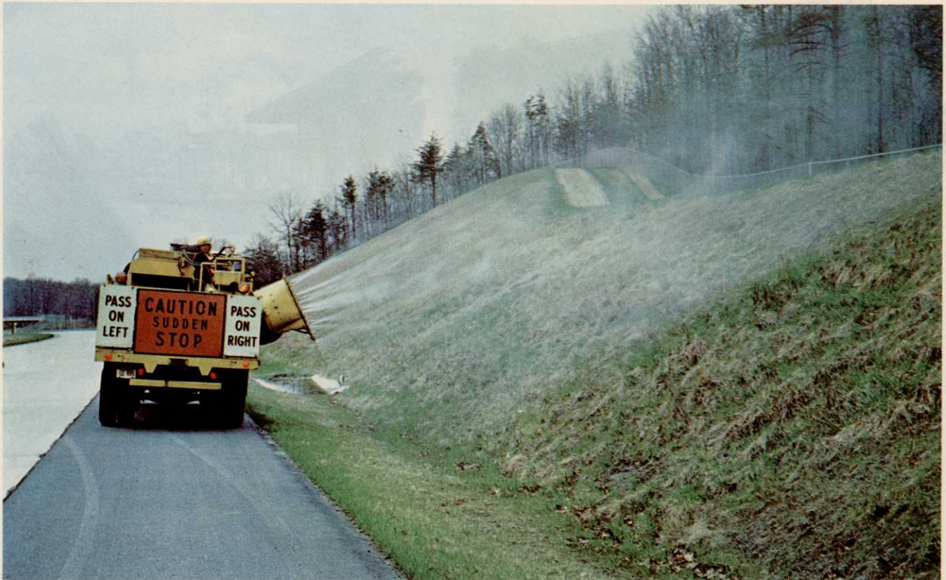
Early spraying with agricultural chemicals on highway rights-of-ways can reduce maintenance costs later in the year. Here, maleic hydrazide, a growth regulator, is being sprayed on slopes to reduce vegetative growth. Highway crews find chemicals eliminate much tedious work.
