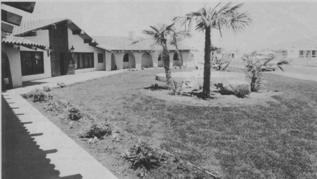
Completed recreation center lawn increases the appeal of the mobile home complex instantly. It takes a crew of three men, working seven hours, to put down approximately 7500 square feet of sod a day.
