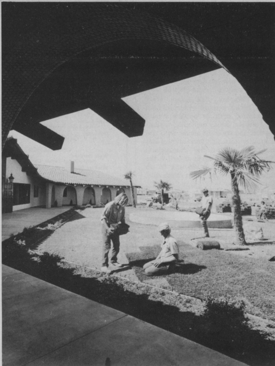
Workmen from Town and Country Landscaping and Supply Company of Los Gatos unroll strips of sod. The bare dirt yard in front of the recreation center at Pacific Western Mobile Estates complex is quickly transformed into lush green grass.
