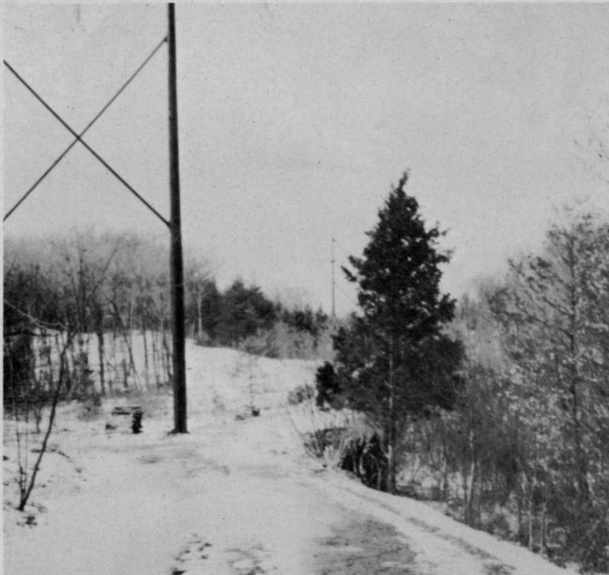
Selective initial clearing for a 345 KV line through a public recreation area includes a narrow access road with small trees and shrubs saved.
