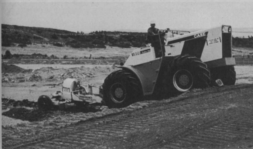
Kessen pipe-puller laying pipe. Puller works from a starter slit trench and pulls pipe through soil without trenching. On some jobs, puller can cut pipe placement time in half when compared to trenching.
