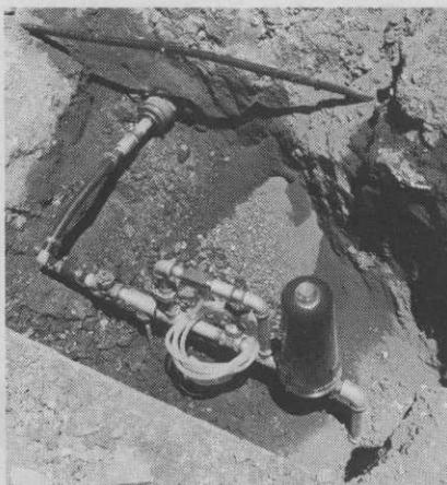
A filter and fertilizer applicator can be integral part of the system.
