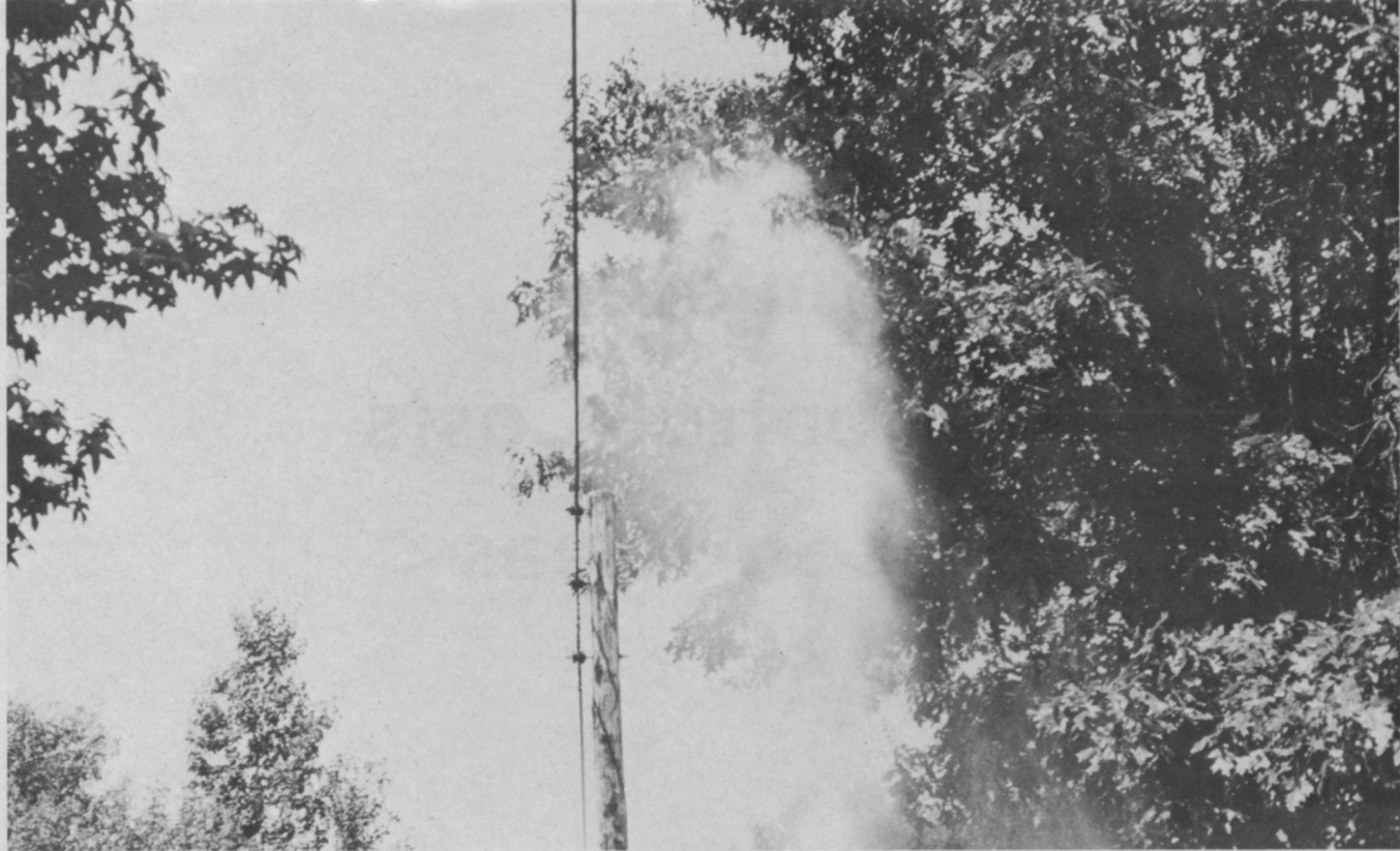
Utility companies are realizing great savings in manpower and dollars by using herbicides to chemically trim trees and brush along rights-of-way. Here, herbicides are sprayed on foliage adjacent to power lines.
