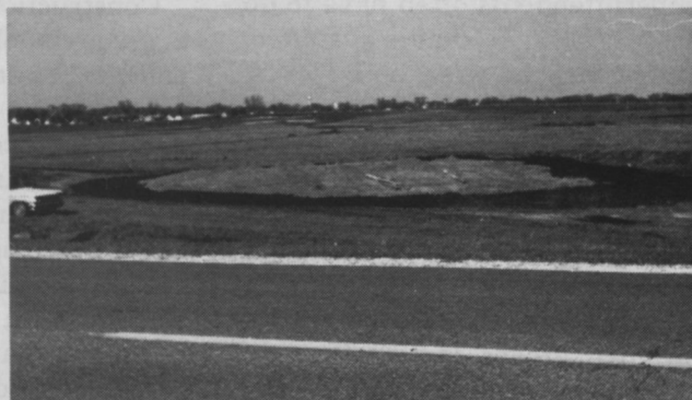
Green site prior to adding mix. Mix is pushed onto site. Heavy equipment is used on green only after buildup of 10 inches or more of topsoil mix.
