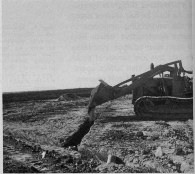
Drainage system is installed prior to forming of basin for green. This important step is often neglected.
