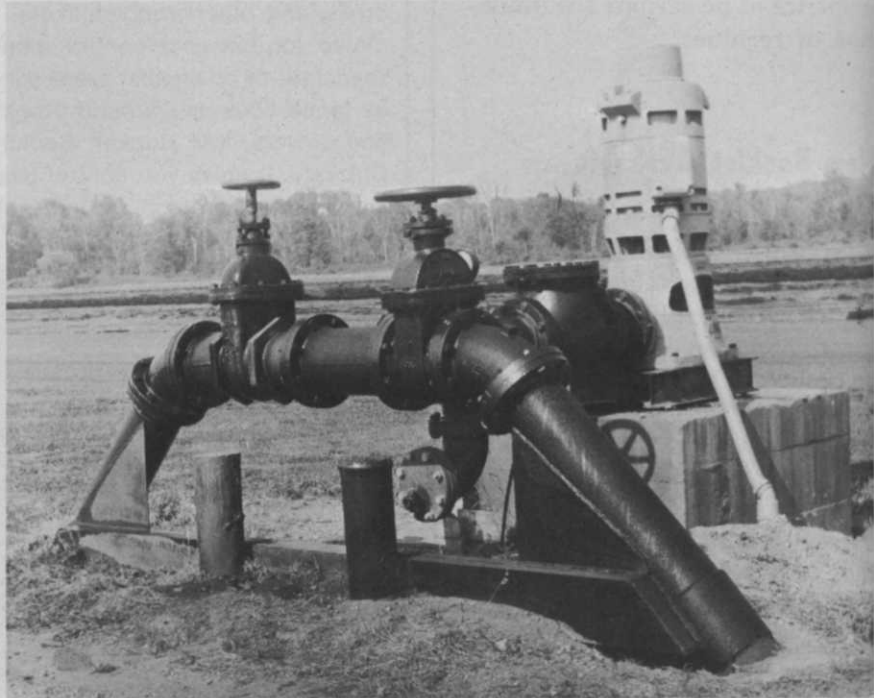
Electrically driven deep well pump is one of 3 used at Emerald Valley Turf Nurseries. Pumps can deliver irrigation water at rate of 2½ million gallons daily. Four miles of 10-inch underground pipe is used to carry supply to quick-coupling surface pipe.
