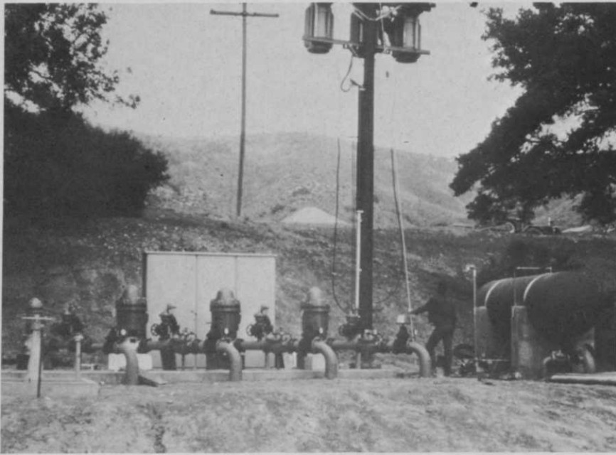
Pumping station on Calabasas Course is capable of supplying 1800 cpm from three 550 gpm pumps and one 150 gpm pump. Pumping units operate on a pressure call or demand system and are lake fed.
