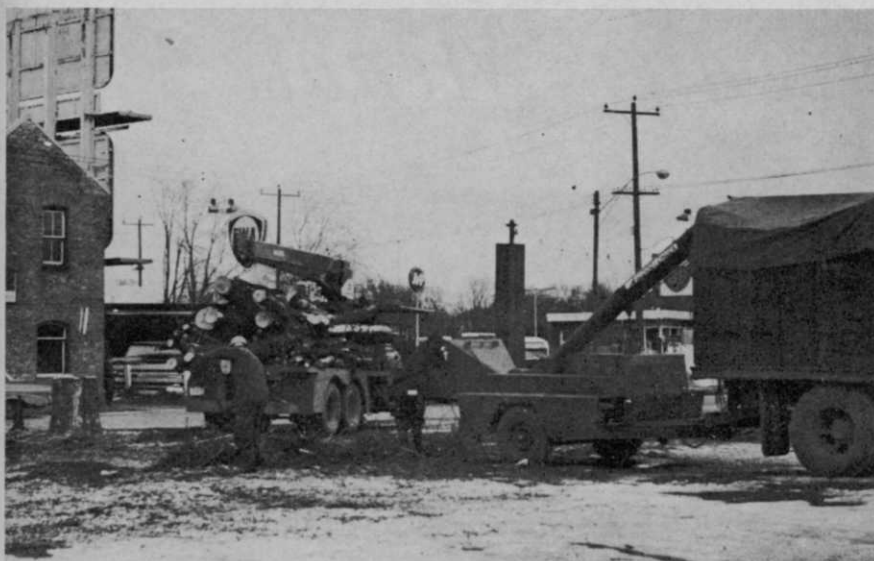
Two men handle removal job in less than 2 hours. Stump, logs, and chips are all that remain of 85-foot tree. Hamilton says mechanized equipment makes this type operation possible.
