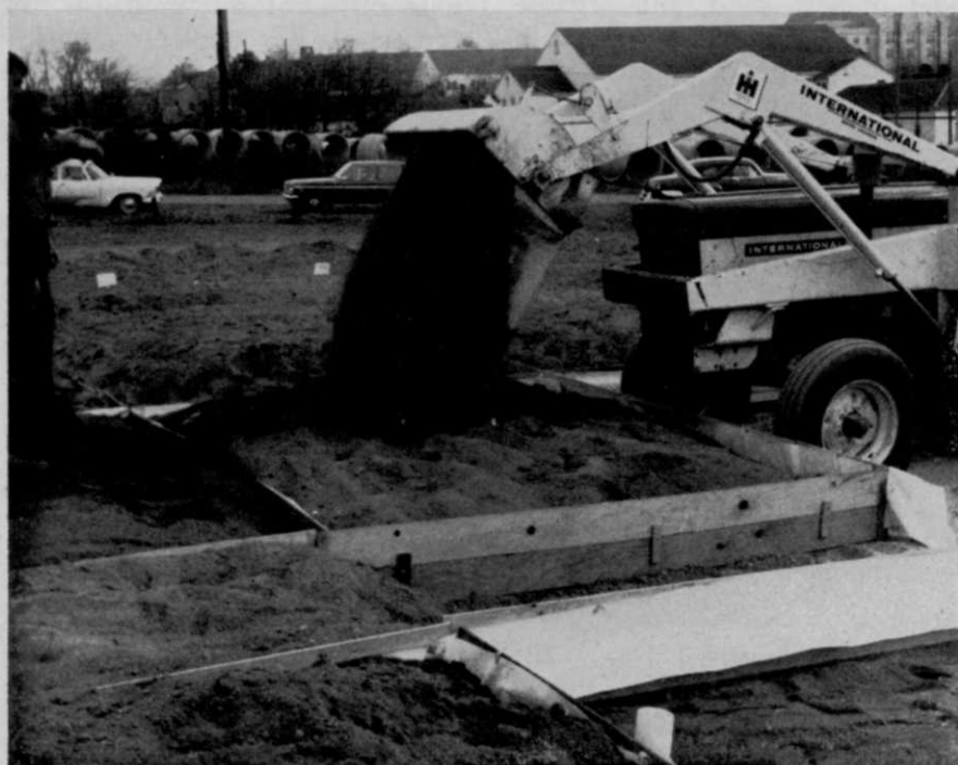
Construction of an experimental putting green at Virginia Polytechnic Institute for evaluating various soil mixtures adaptable to today's heavy golf traffic.
