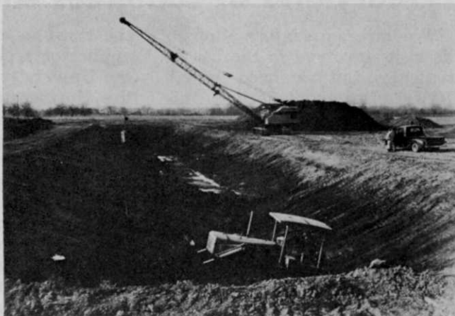
Drainage ditch being cut (right) will flow into one of three reservoirs. All work except heavy excavating is done by Mercer.
