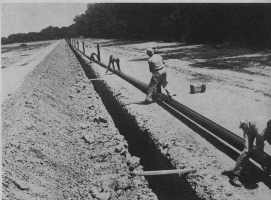
Workmen prepare to lower a section of eight-inch aluminum water main, which is part of Summit Hall's permanent irrigation system. When completed, the system will be one of the largest of its kind in the country.
