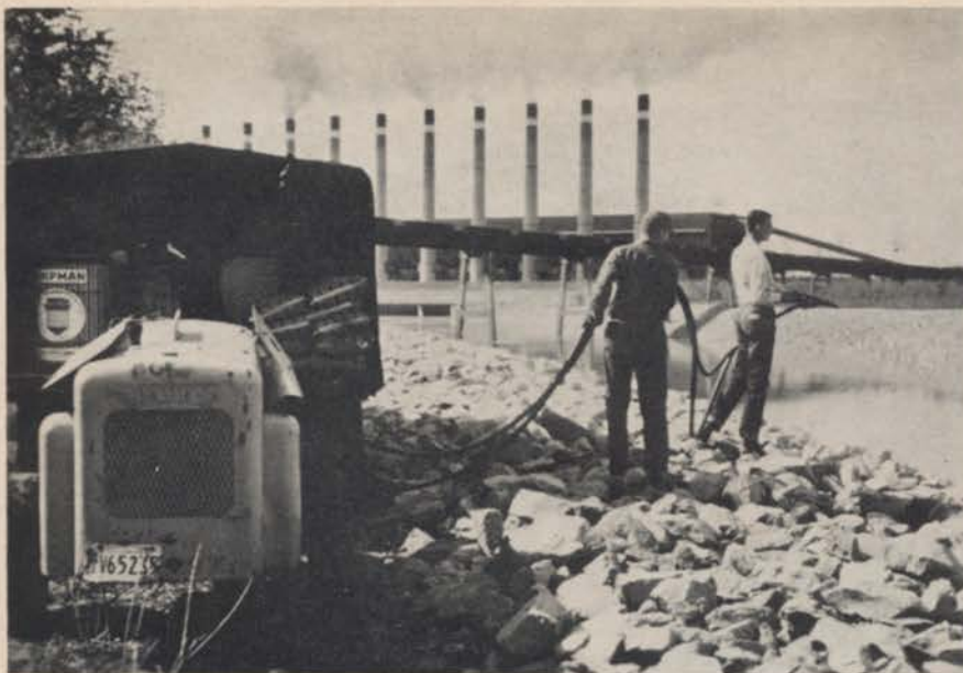
Around steam plants, such as these, TVA workers prefer to use soil sterilants to effect weed control.
