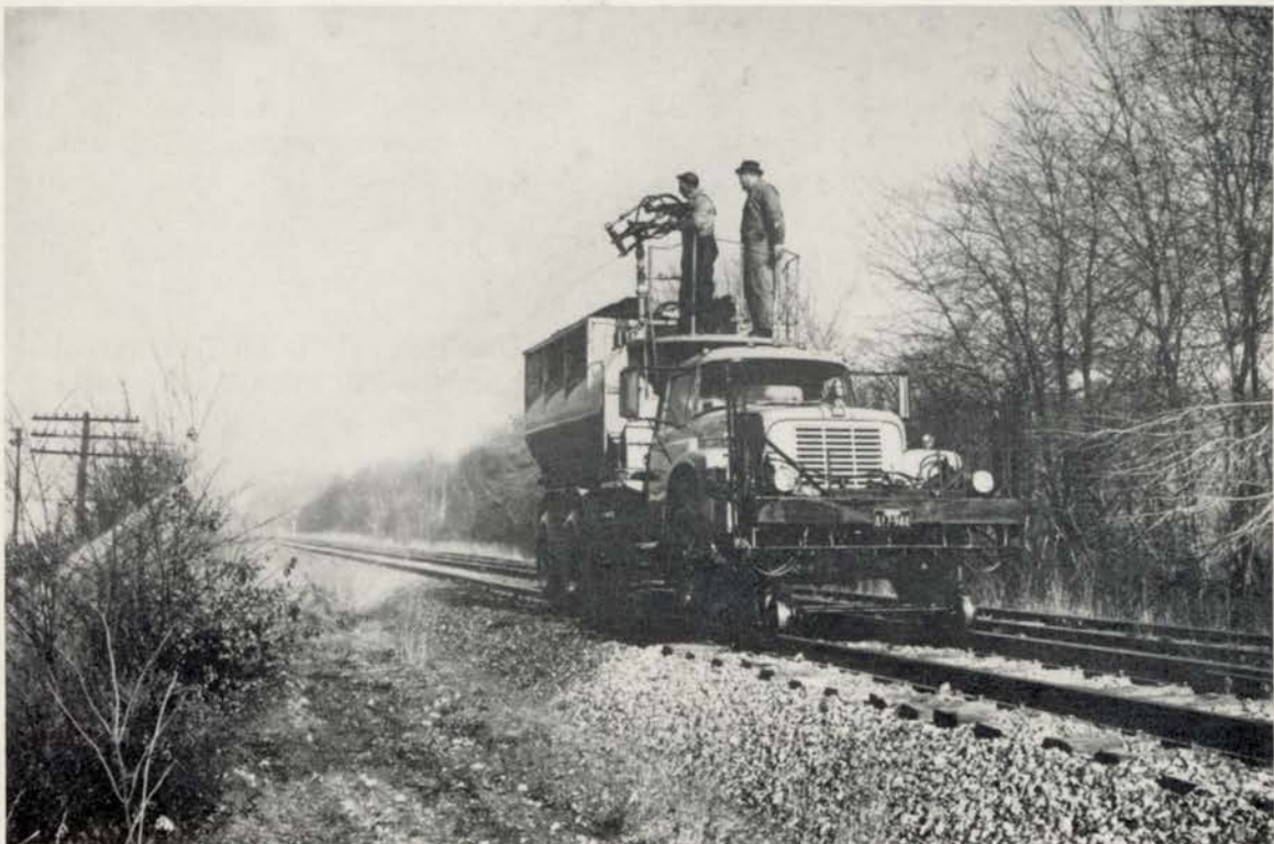
Spraying rights of way for brush control during dormant season is receiving widespread attention.
