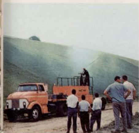
1. Turfiber being sprayed on 3:1 slope along New Jersey interstate highway project. Two days later, hurricane Donna dumped five inches of rain on the Turfiber treated area.
