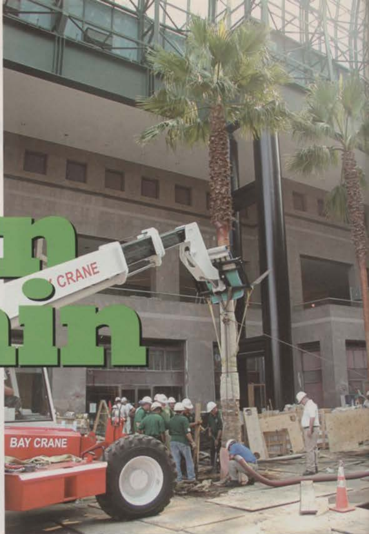
The most efficient way to plant the 40-ft. palms was to use a crane to ease them into planting chambers, then blow the specially blended soil around the roots.
