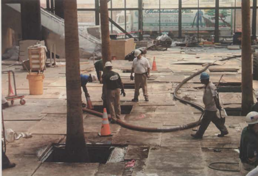
The Winter Garden restoration project at the World Financial Center was accomplished through the coordinated efforts of many different tradesmen.
