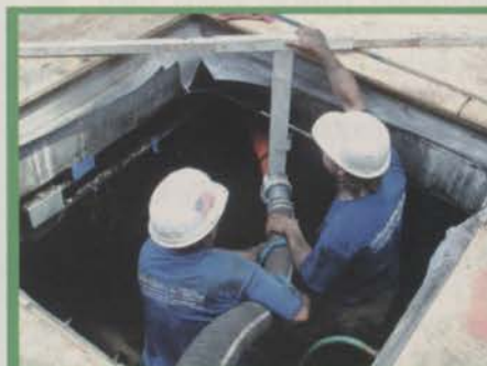
Mulchmaster workers blew a layer of round gravel for drainage into the planting hole first.
