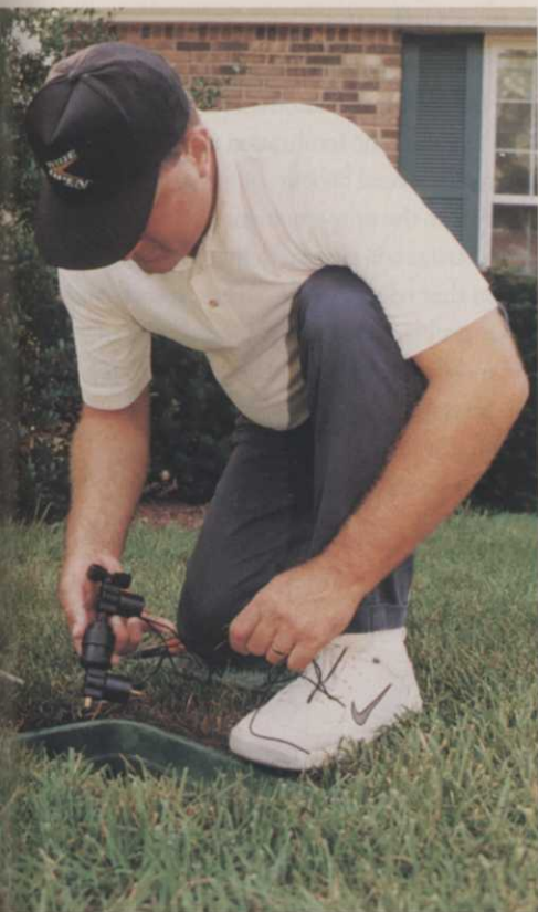
Installation and maintenance of residential fertigation systems is relatively simple.
